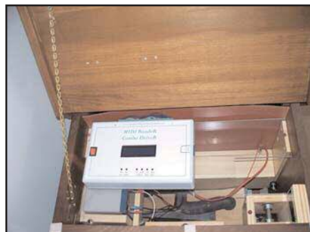
Figure 2. The new MIDI unit installed.
